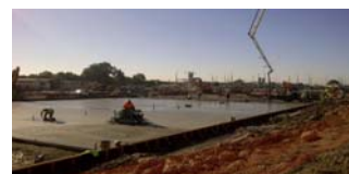
Construction work on Emporium Melbourne, Vic (Top) Works underway at Roxburgh Park, Vic (Bottom)
